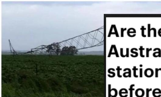
▲ Transmission towers carrying power lines toppled by high winds near Torrens Island, South Australia. Debbie Prosser/AP/Getty Images
