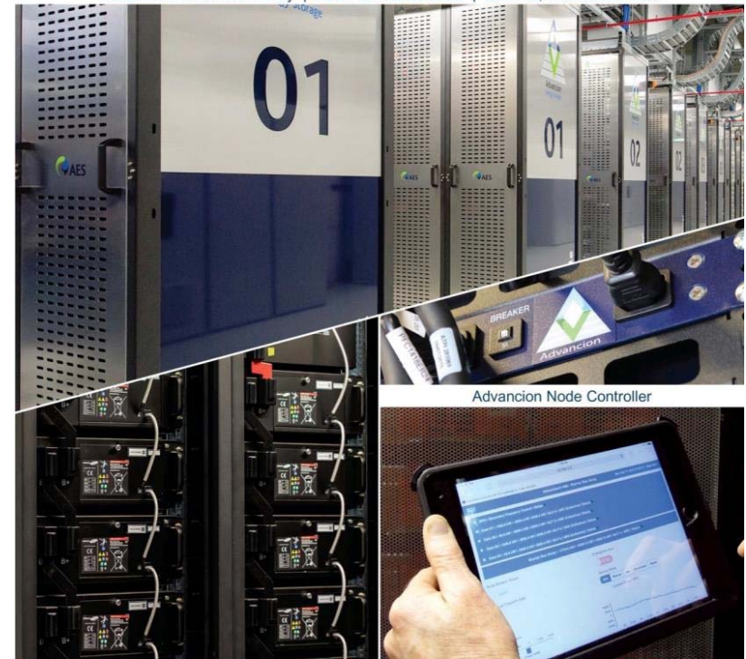
Batteries in a Advancion Node
