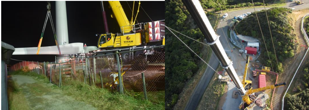
Figure 6: The new Brooklyn Turbine under construction in 2016. Note the predator proof fence in the left of the left-hand photo and on the right of the right-hand photo. The Brooklyn Turbine is right next to the most significant bird sanctuary in New Zealand.
