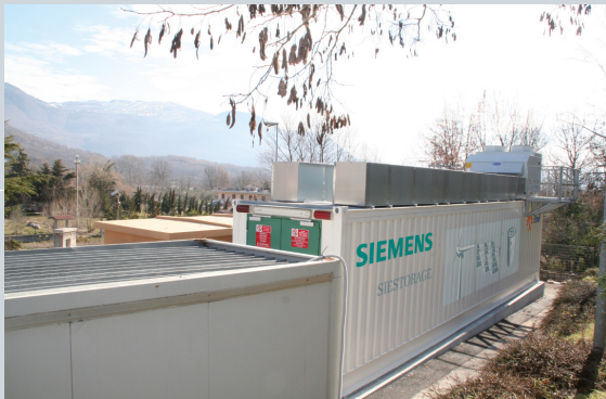
SIESTORAGE installation at the grid of ENEL (Italy's largest energy supplier) – Installation and commissioning 2012 – 1MVA/500 kWh
